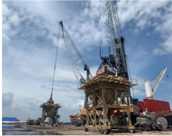
View of the Equipment located within Berth 9
